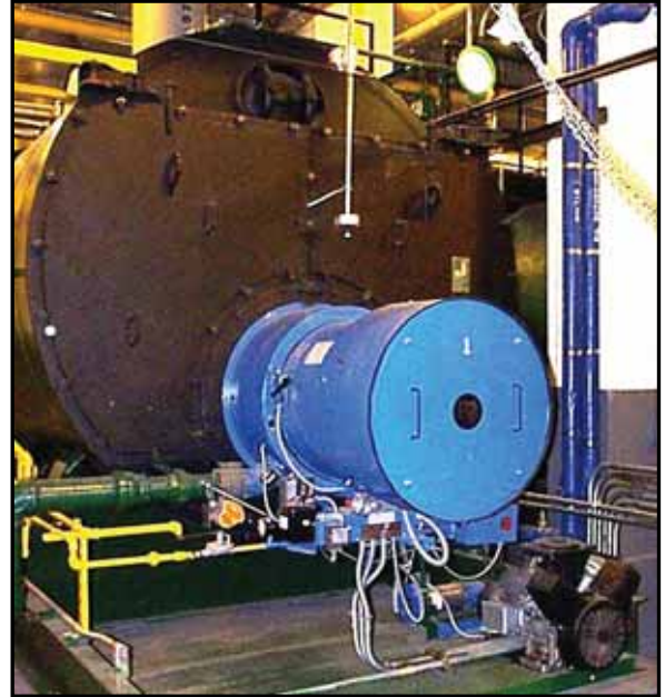
FD68CA400LM installed on a new packaged boiler system.
